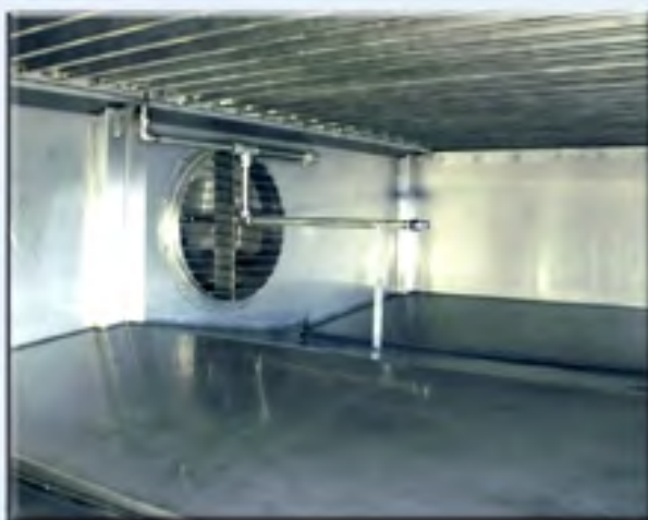
TYPICAL CLEAN INTERNAL DESIGN
